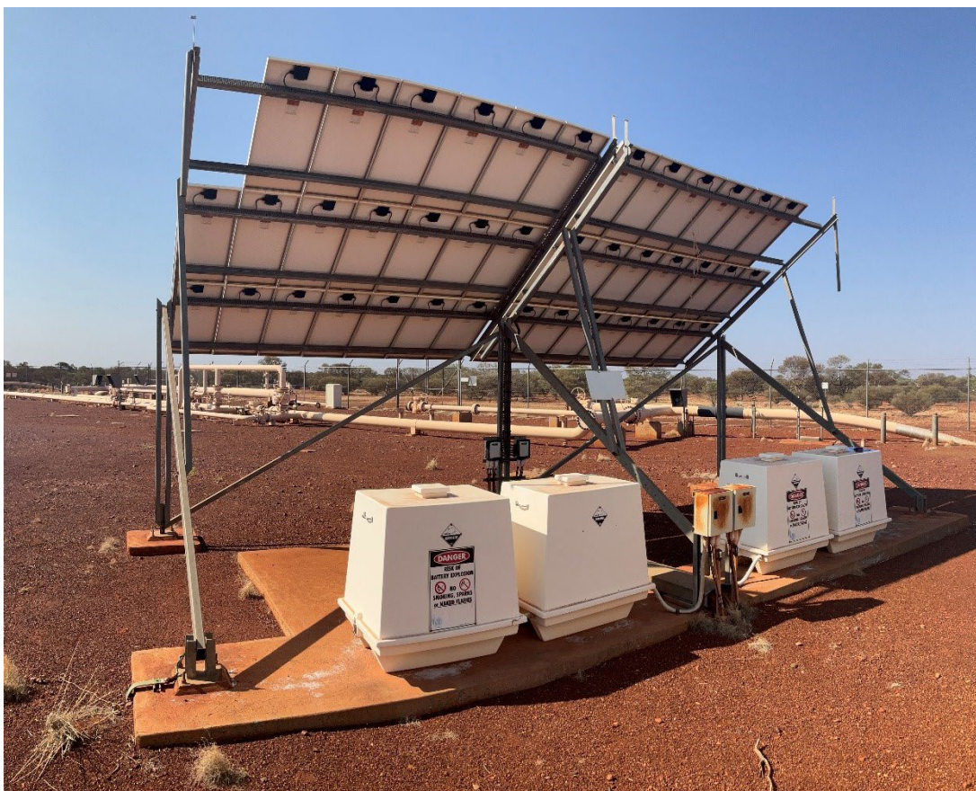
Figure 4 Newman Scraper Station Power system
