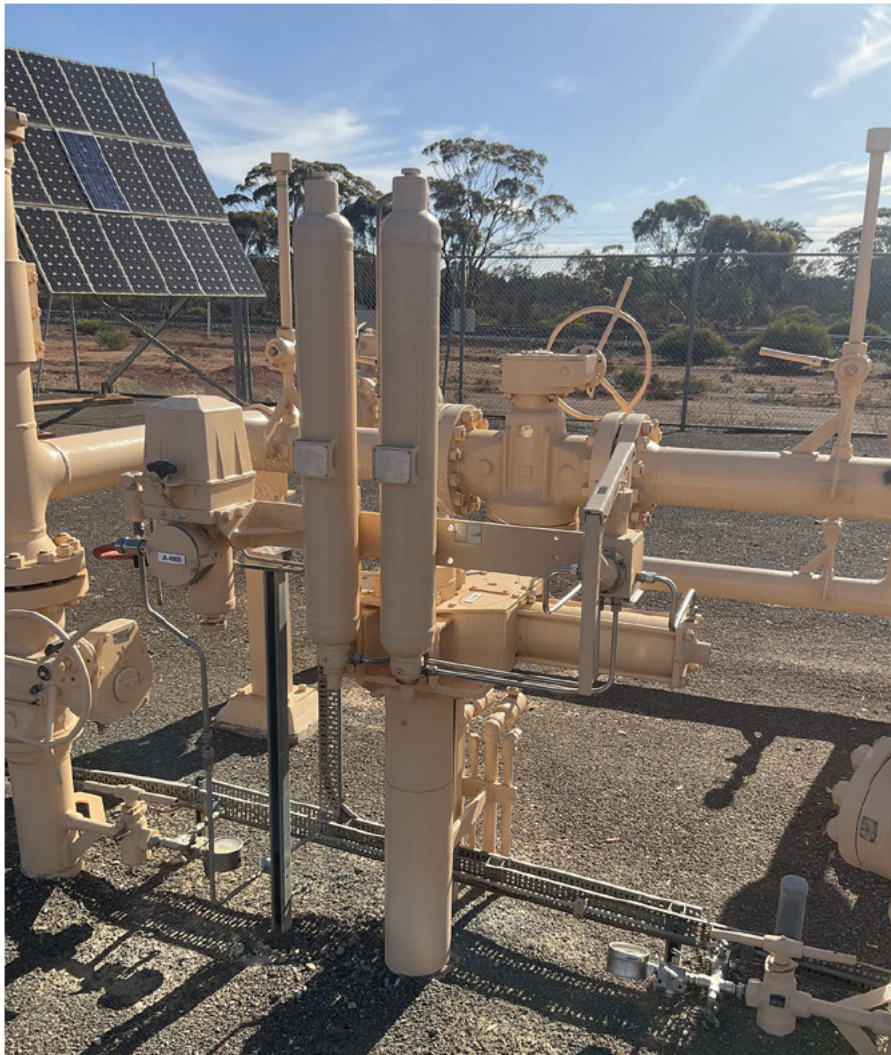
Figure 3 Kalgoorlie North Main Line Valve
