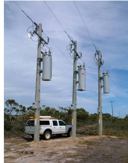
Distribution automation devices
