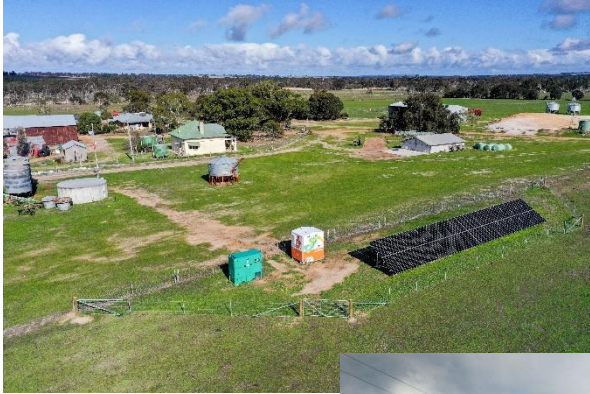
Standalone power system (SPS)
