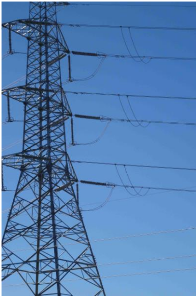
Paralleling to energise other circuit
