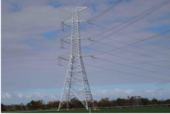
Tower for future connection for Golden Grove
