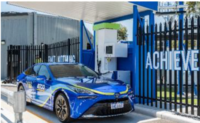
Figure 6: Hydrogen Refueller at ATCO's Jandakot facility
